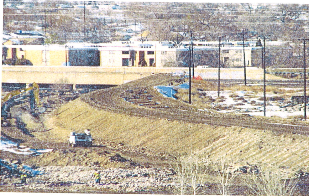
Levee work looking NW from Dutch Clark Stadium Crushing operation is located in lower left; Access ramp to the top of the levee lower right. Slopes are being rough graded and the top of the Levee is being graded for the maintenance road. Picture was taken on January 22 nd .
