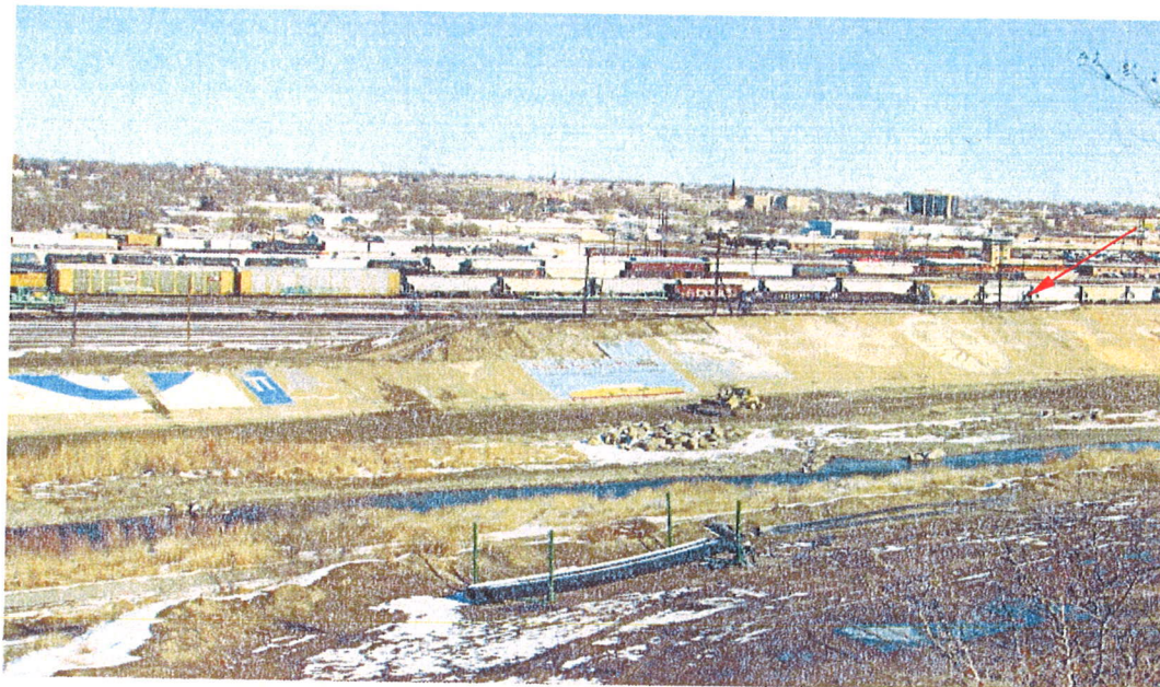
Levee work looking SE from Dutch Clark Stadium This picture was taken on January 22 nd showing the progress near the end of Phase I (red arrow). The bottom of the levee has been graded along the toe in preparation for the work in the river.
